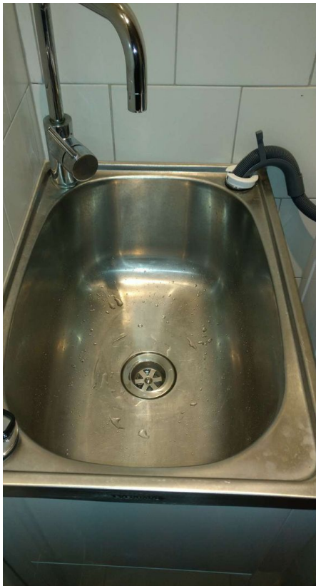
Laundry Tub/Sink Condition: In serviceable condition at the time of inspection
